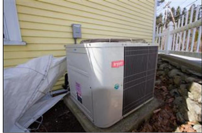
9.8 Picture 2 AC Condenser
