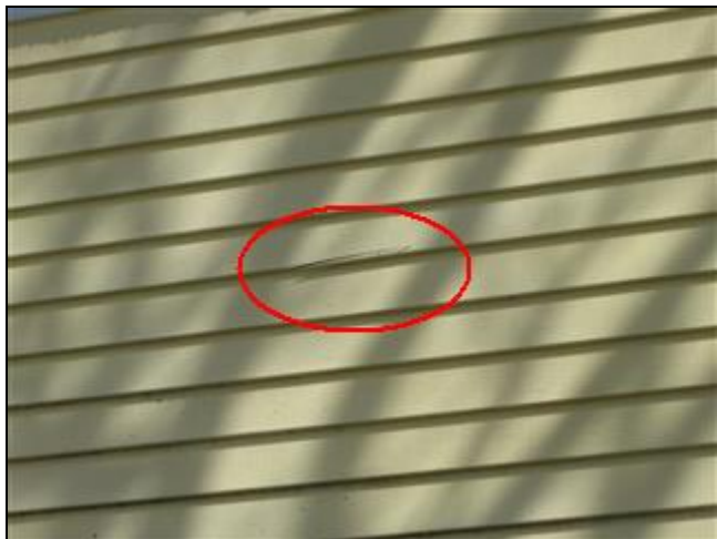
2.0 Picture 1 Cracked clapboard
