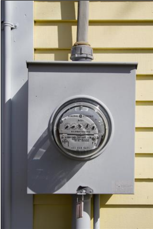
8.1 Picture 1 Service Meter
