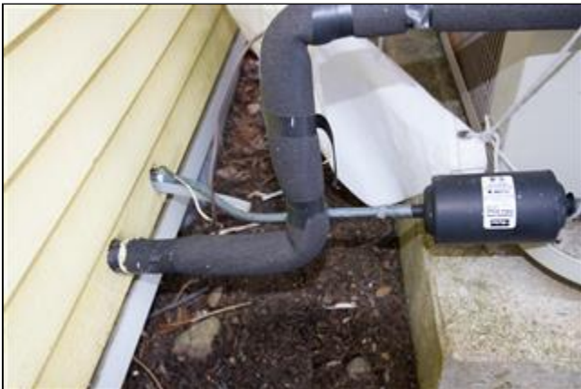
9.8 Picture 3 AC Condenser
