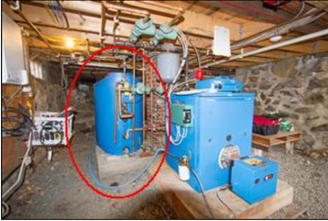
7.2 Picture 1 Hot Water Tank
