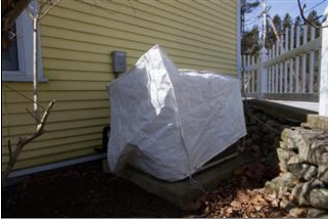
9.8 Picture 1 AC Condenser
