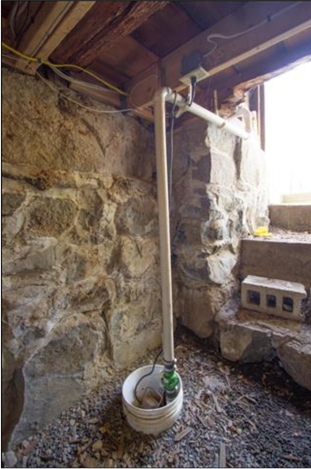
7.6 Picture 1 Sump Pump South
