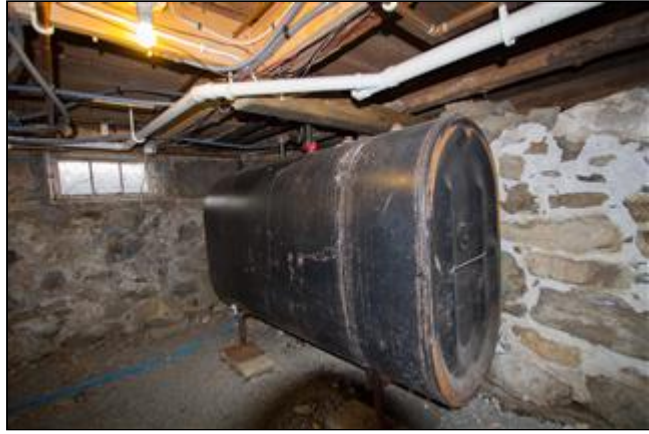
7.4 Picture 1 Oil Tank
