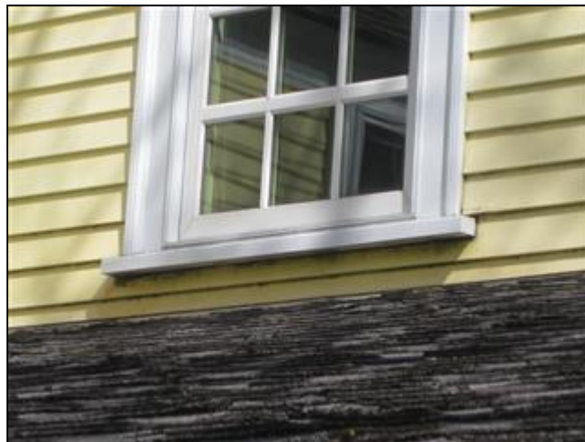
2.0 Picture 2 Dirty cladding
