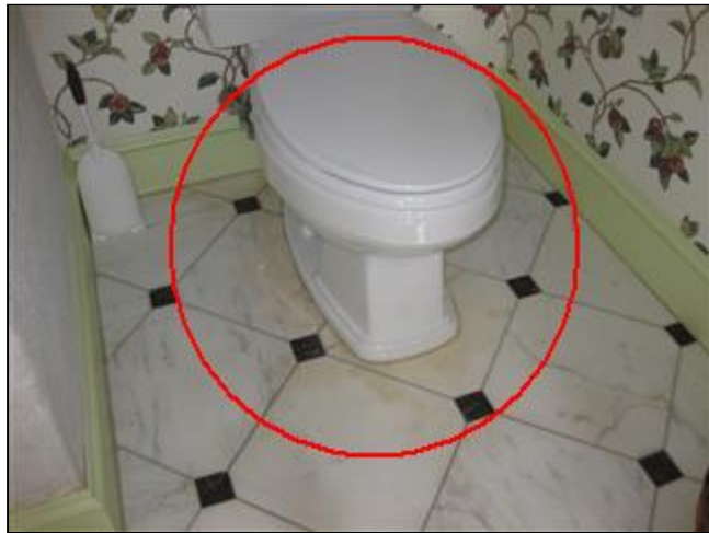
5.4.B Picture 1 Toilet Stains
