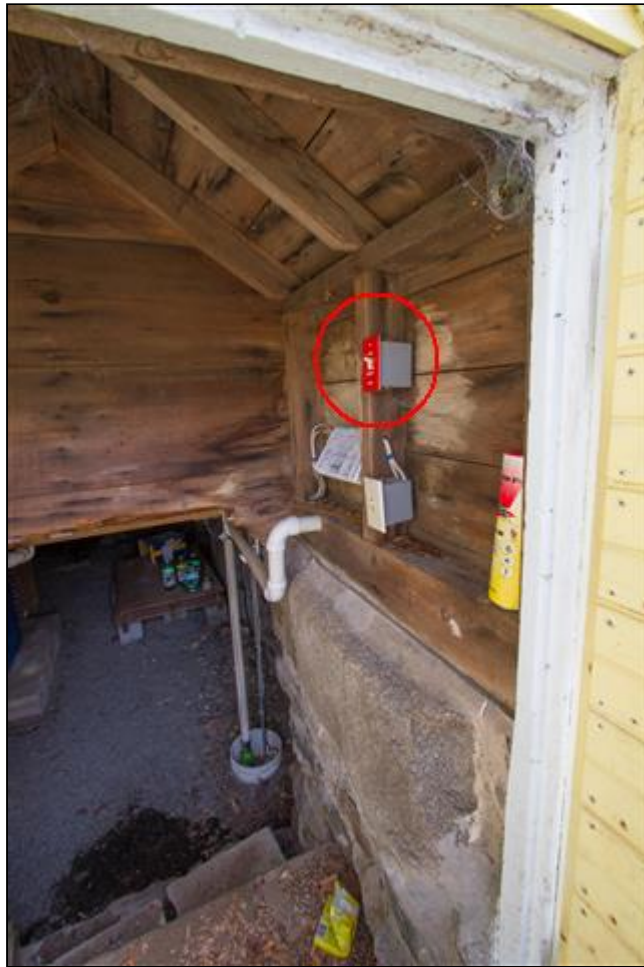
9.2 Picture 1 Boiler Safety Switch
