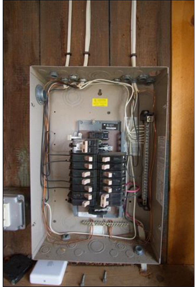
10.8 Picture 2 Sub Panel
