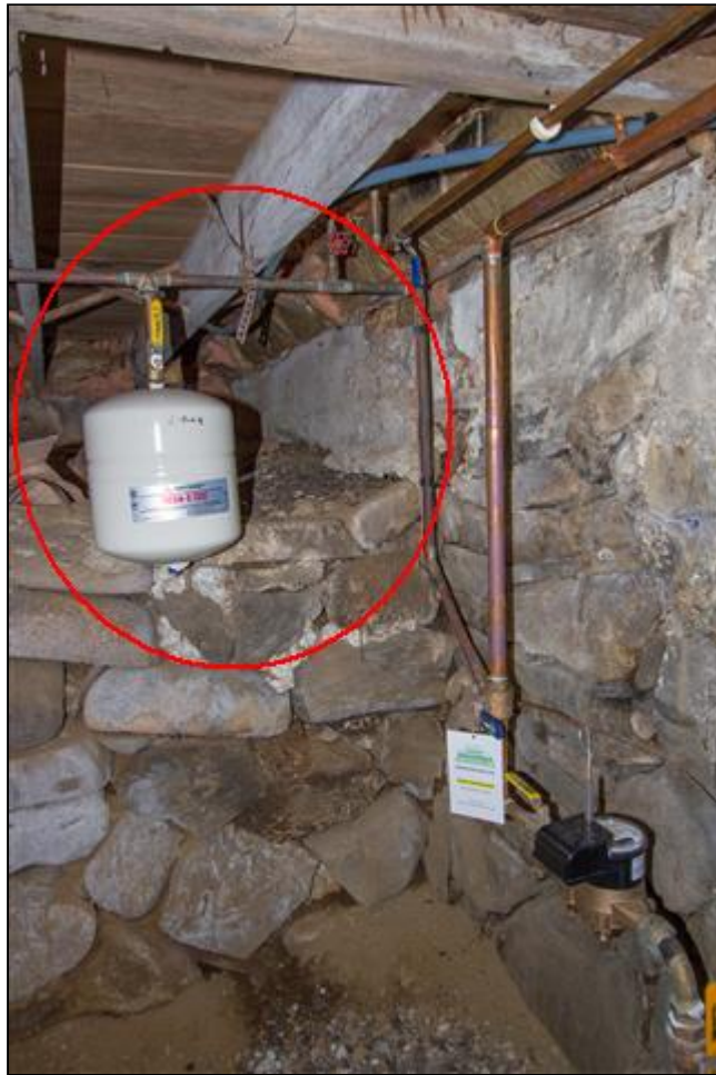
7.1 Picture 1 Expansion Tank
