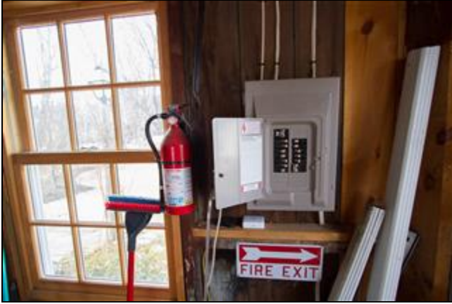
10.8 Picture 1 Sub Panel
