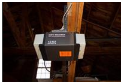
10.11 Picture 1 Garage Door Operator
