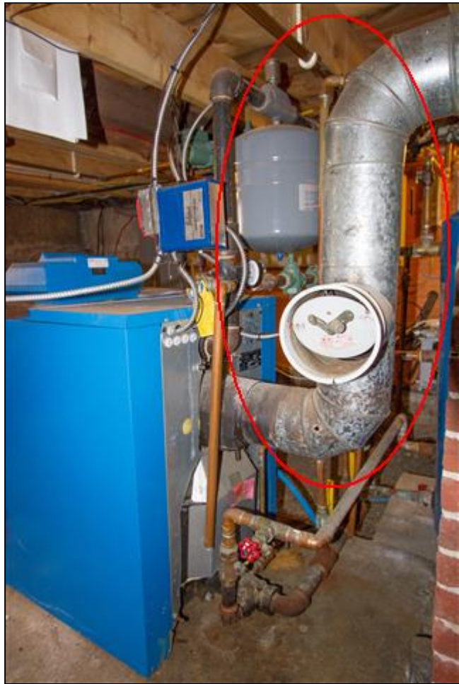
9.5 Picture 1 Boiler Flue
