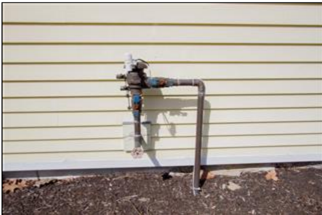
7.3 Picture 1 Exterior Shut Off
