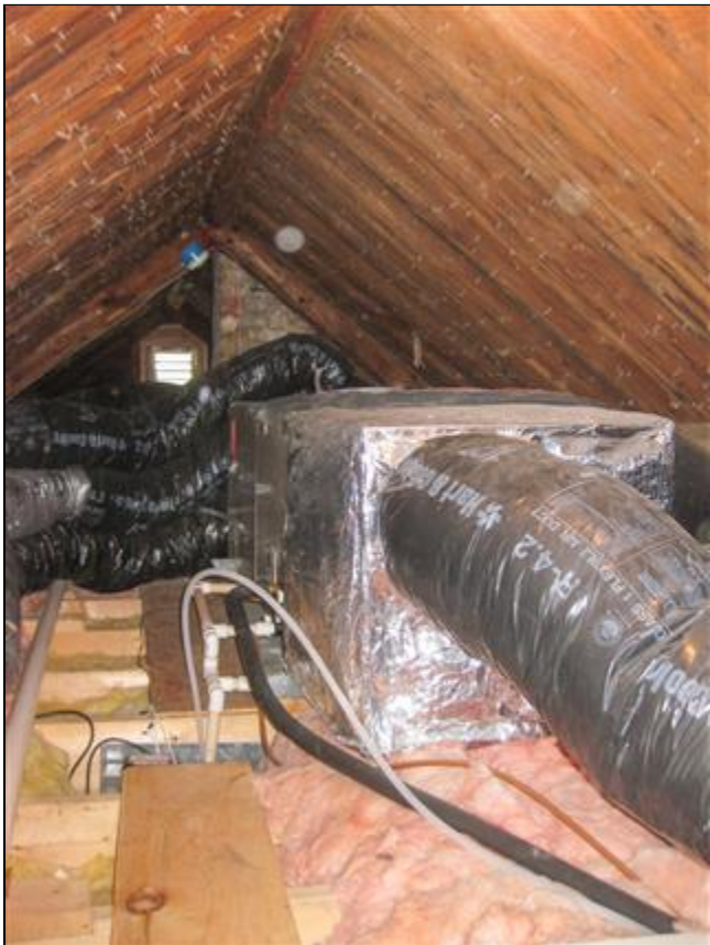
9.8 Picture 5 A/C Air Handler
