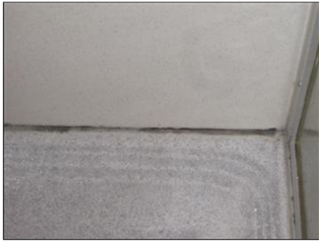
5.4.A Picture 1 Shower Sealant.
