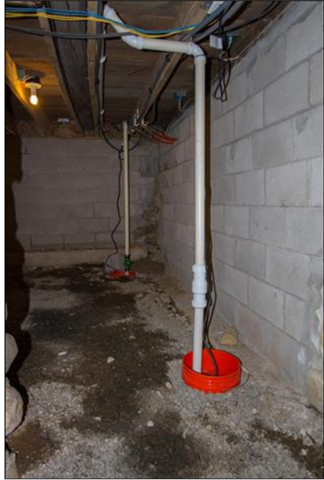
7.6 Picture 2 Sump Pumps East
