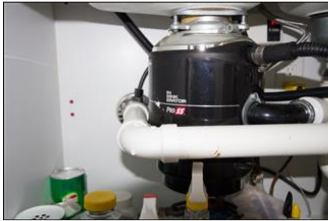
3.14 Picture 1 Garbage Disposal
