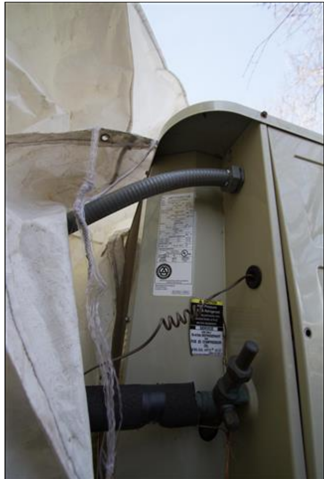
9.8 Picture 4 AC Condenser
