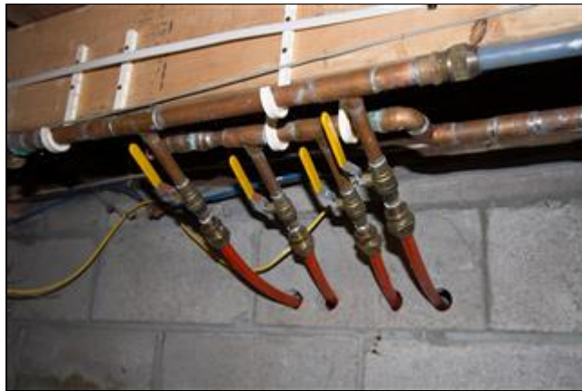
9.3 Picture 1 Radiant Heat valves
