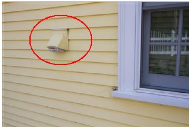
3.16 Picture 1 Dryer Vent
