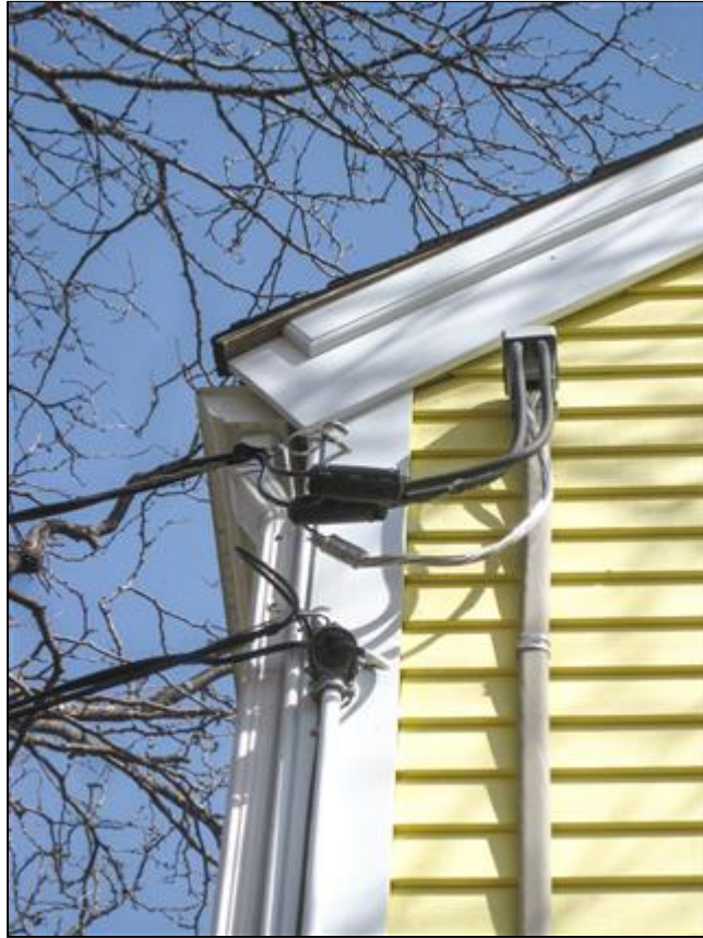
8.0 Picture 1 Service Entrance Conductors
